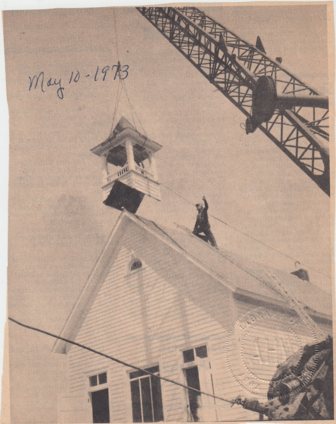
The bell tower on the restored rural school in Pine City was placed back into position Tuesday afternoon and the old structure once again took on its proper country school appearance. The big crane from Rydberg Construction gently set the ornate tower back on its lofty perch. Volunteer labor will now be needed to finish the interior painting so the school can open for public viewing this summer.
